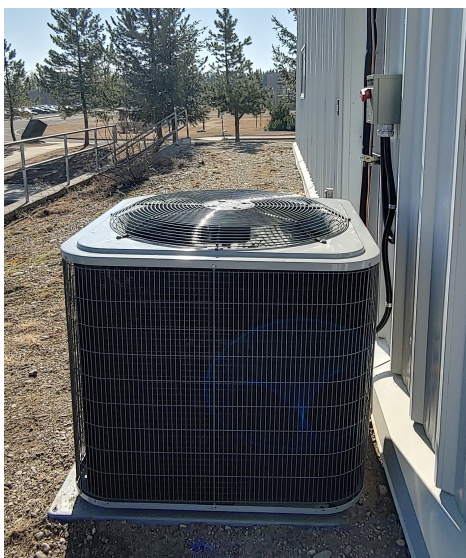
Figure 2: Maintenance Building Heat Pump
