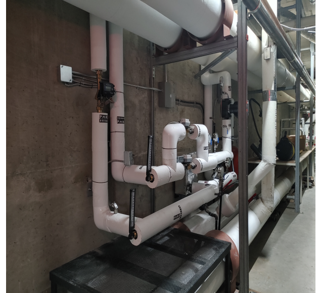
Figure 1: Upgraded Agora Heat Exchanger System
