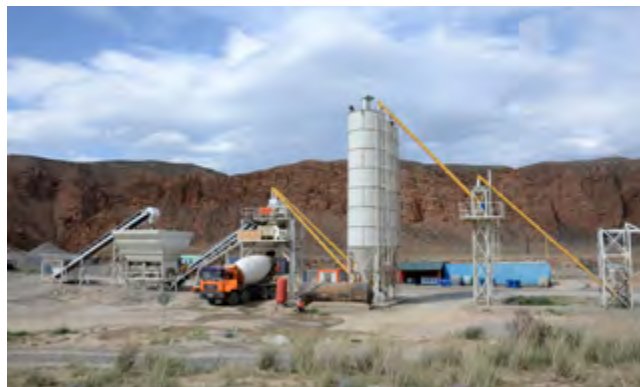
Cement batching plant in Naryn
