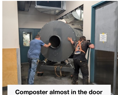
Composter almost in the door to the recycling room.
